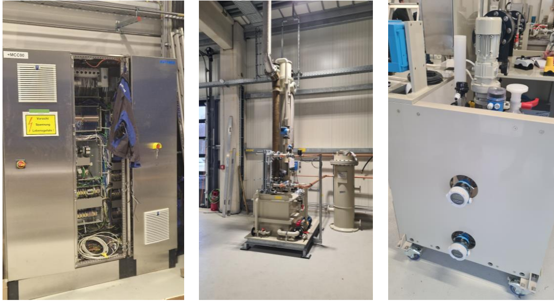
Figure 4 – Electrical Board and Various Equipment
