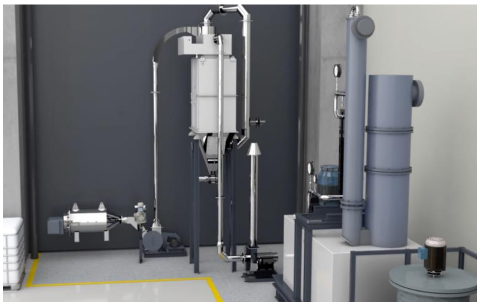
Figure 5.5: Pilot Plant equipment
